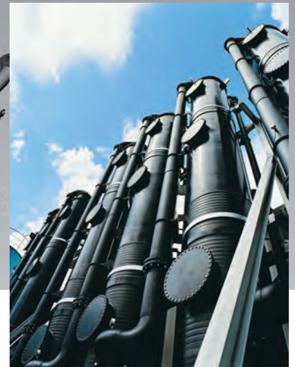
Two-stage desorption column with downstream air activated-carbon filters
